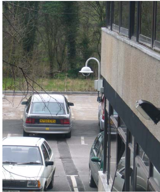
Shand House CCTV Installed under Part 33 of the GPDO
